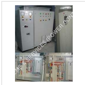
AC And DC Drive Panel
