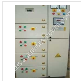
Automatic Power Factor Correction
